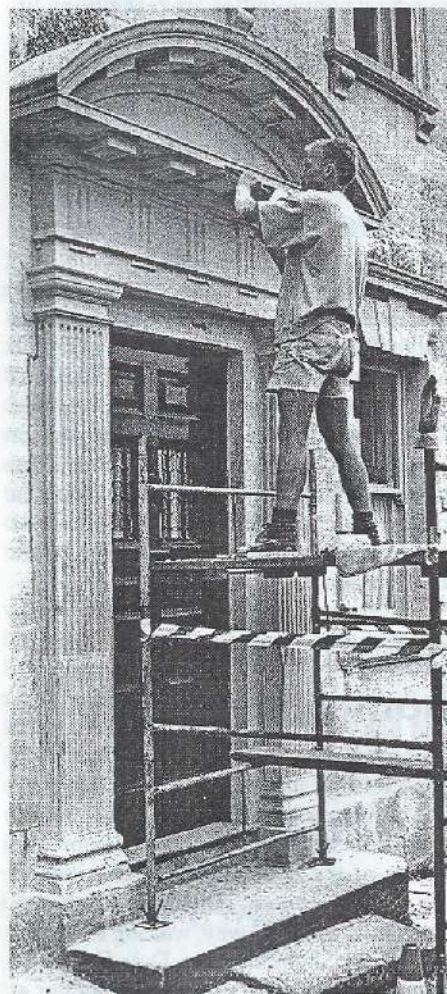
Stonemason Max Knowles at work restoring some of the intricate carving above the entrance to Lovedays House.
